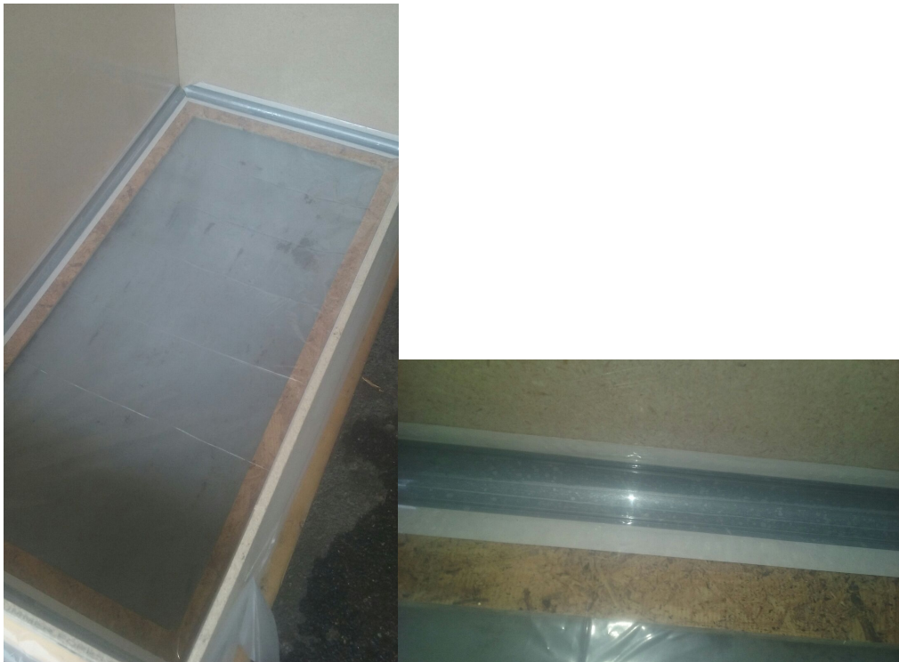
Figure 4: Round corner molds that are typically used in drywall applications, and we used it and taped it in the corners to have a molding part with no sharp edges.
